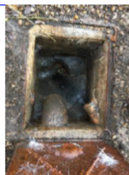
Existing Foul Connection
